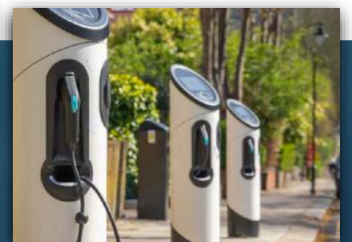
EV Charging Points
